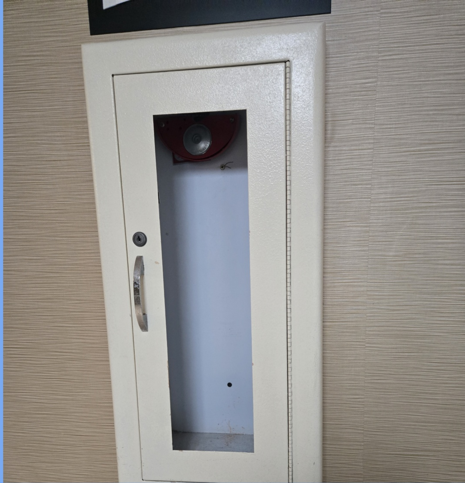
Missing Fire Extinguisher
