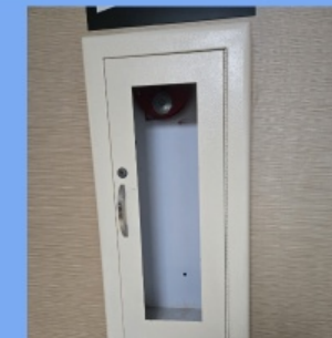
Missing Fire Extinguisher
