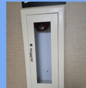
Missing Fire Extinguisher
