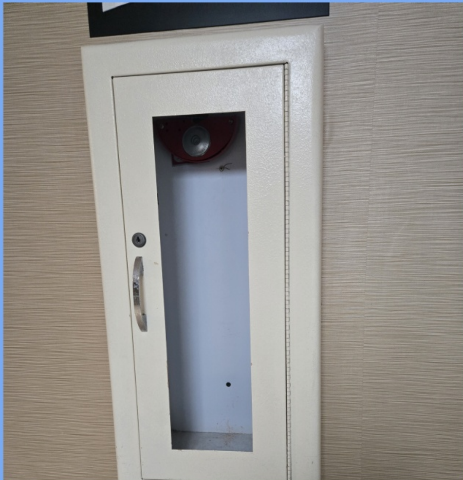
Missing Fire Extinguisher
